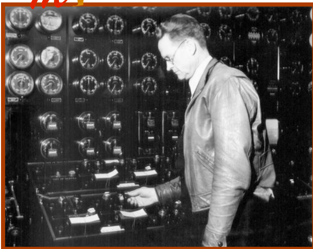
J. A. Griffiths opens the circuit breaker on the last DWP 50 cycle circuit. Taken in the old control house at Receiving Station-C (RS-C).
