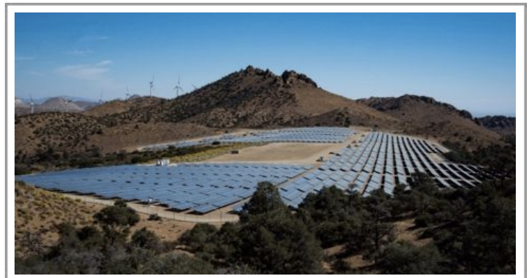
Pine Tree solar panels
