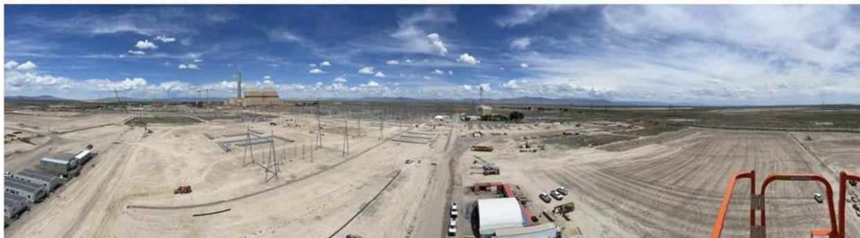
IPP Switchyard Expansion
