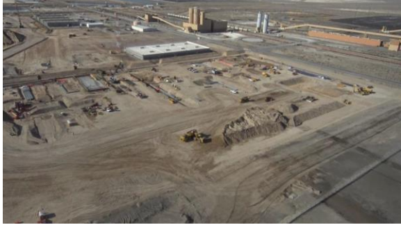
IPP Gas Generator Site November 2022
