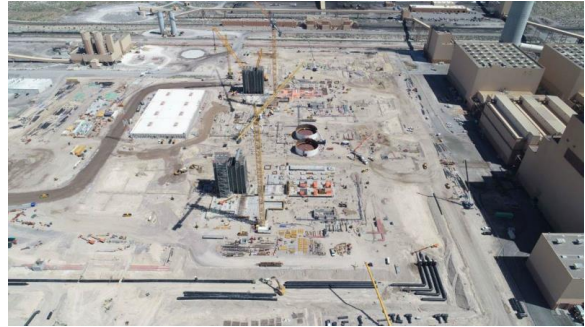
IPP Gas Generator Site June 2023
