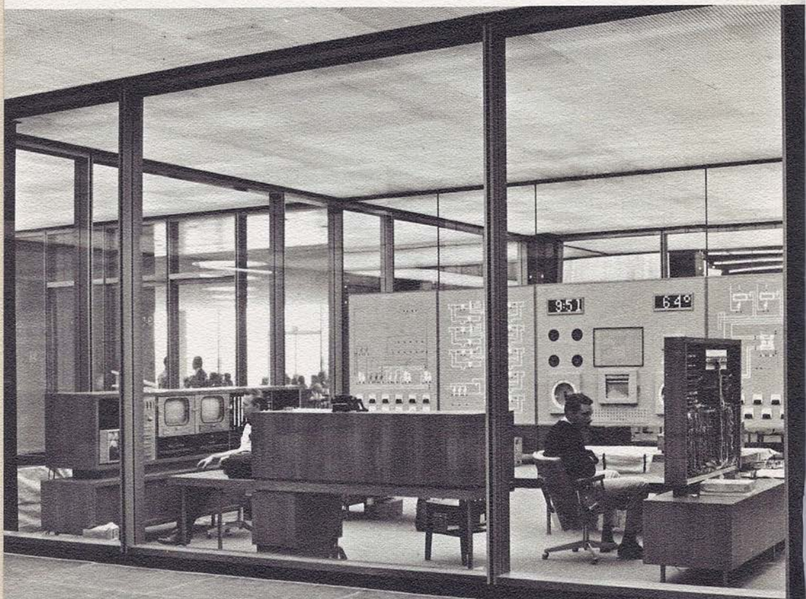
The building's electrical and mechanical equipment is controlled here
