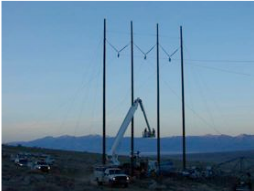
Temporary 4-Pole Wood Structure with V-String Hardware
