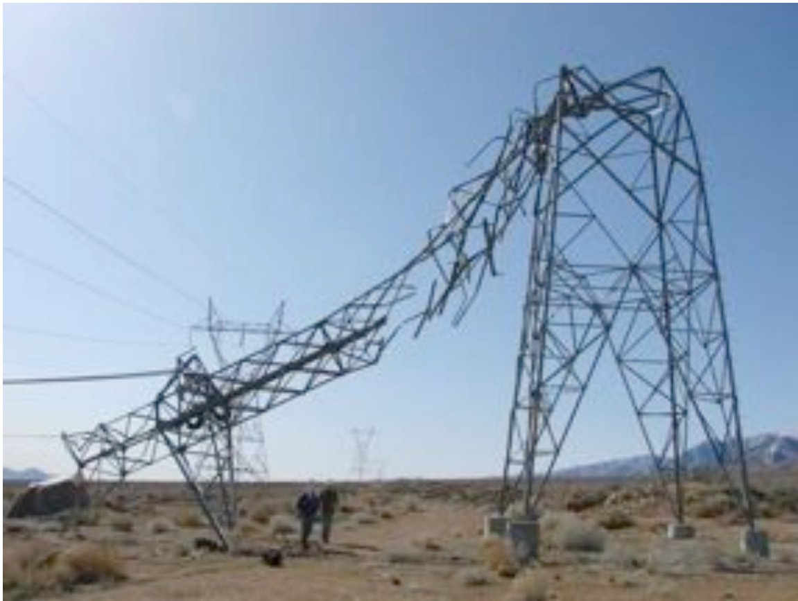
DC Line ISH Tower Failure due to 100+ MPH Winds
