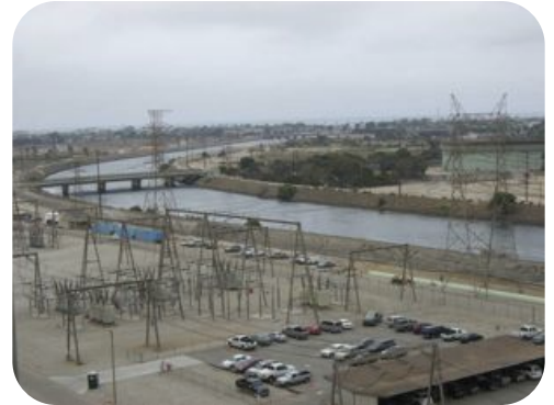
Haynes switchyard next to the San Gabriel River.
