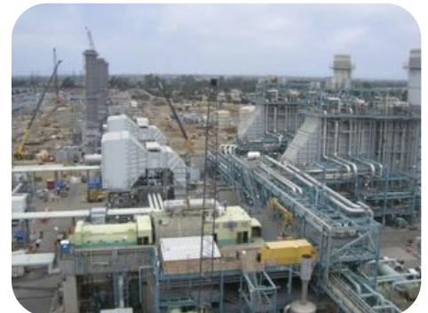
View of 100 MW units as turbine units with the larger combined cycle units to the right.
